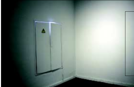
sparking fuse box
